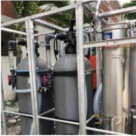
Water Filtration Unit
